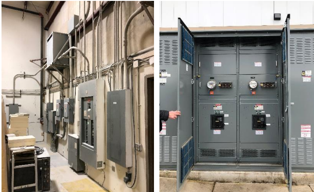
Figure 16: Older interior switchgear with subpanels versus newer onsite switchgear with tenant utility meters.
