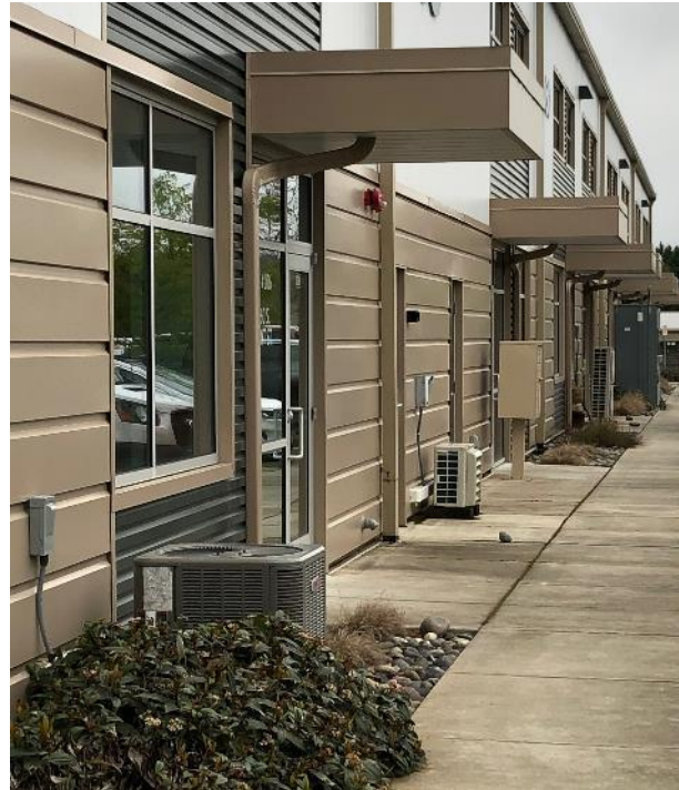
Figure 10: Heat pumps are already common for office spaces in newer light industrial buildings at the Port. These outdoor units show a diversity of equipment performance.
