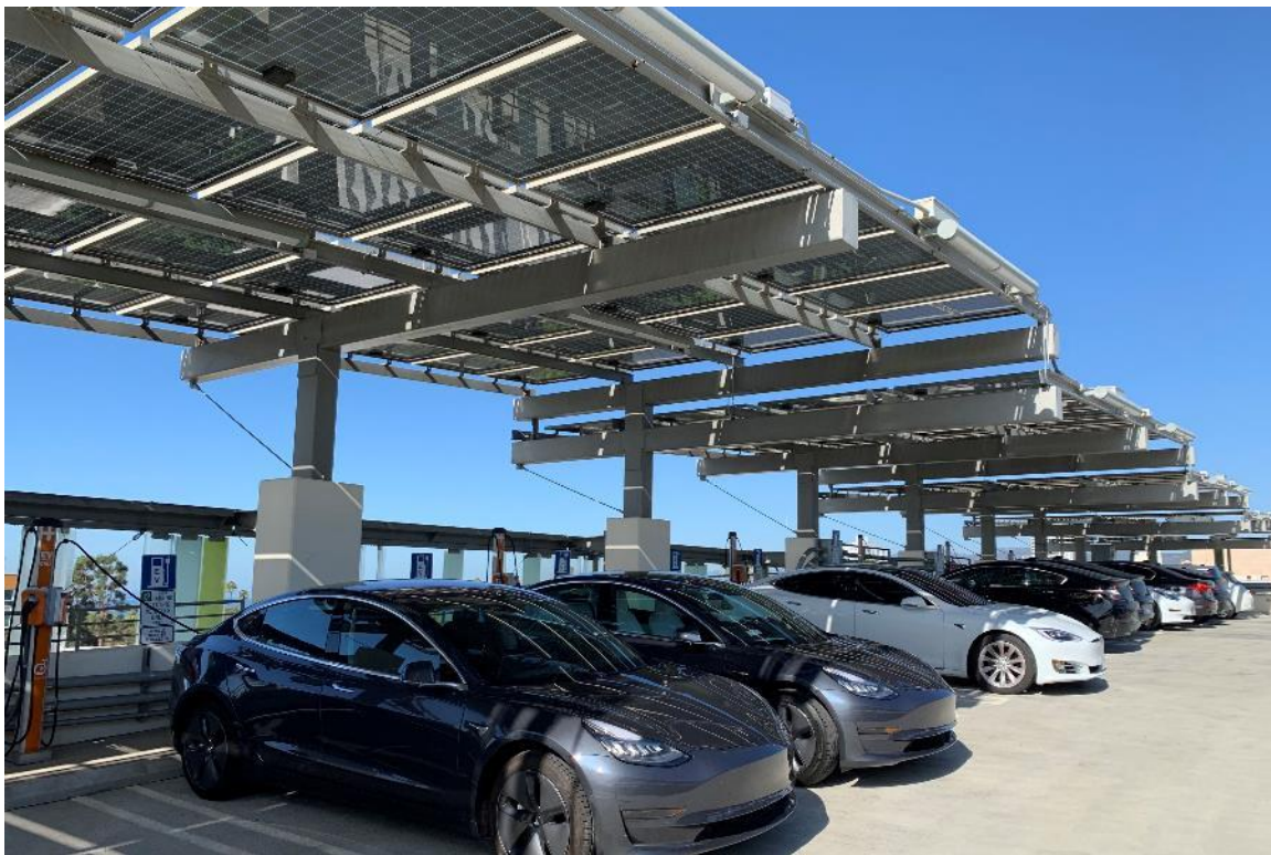
Figure 24: Parking, EV charging and onsite PV can be implemented together. EV charging at the Civic Center Parking Structure in Santa Monica (Courtesy of City of Santa Monica).
