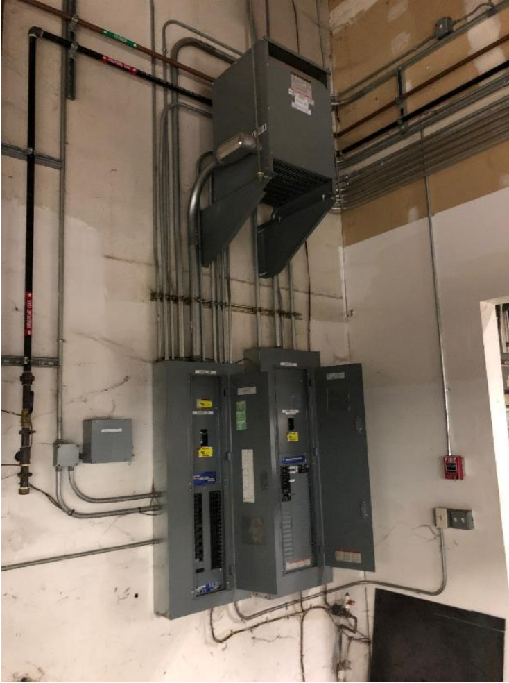
Figure 9: Example of existing onsite electrical infrastructure.
