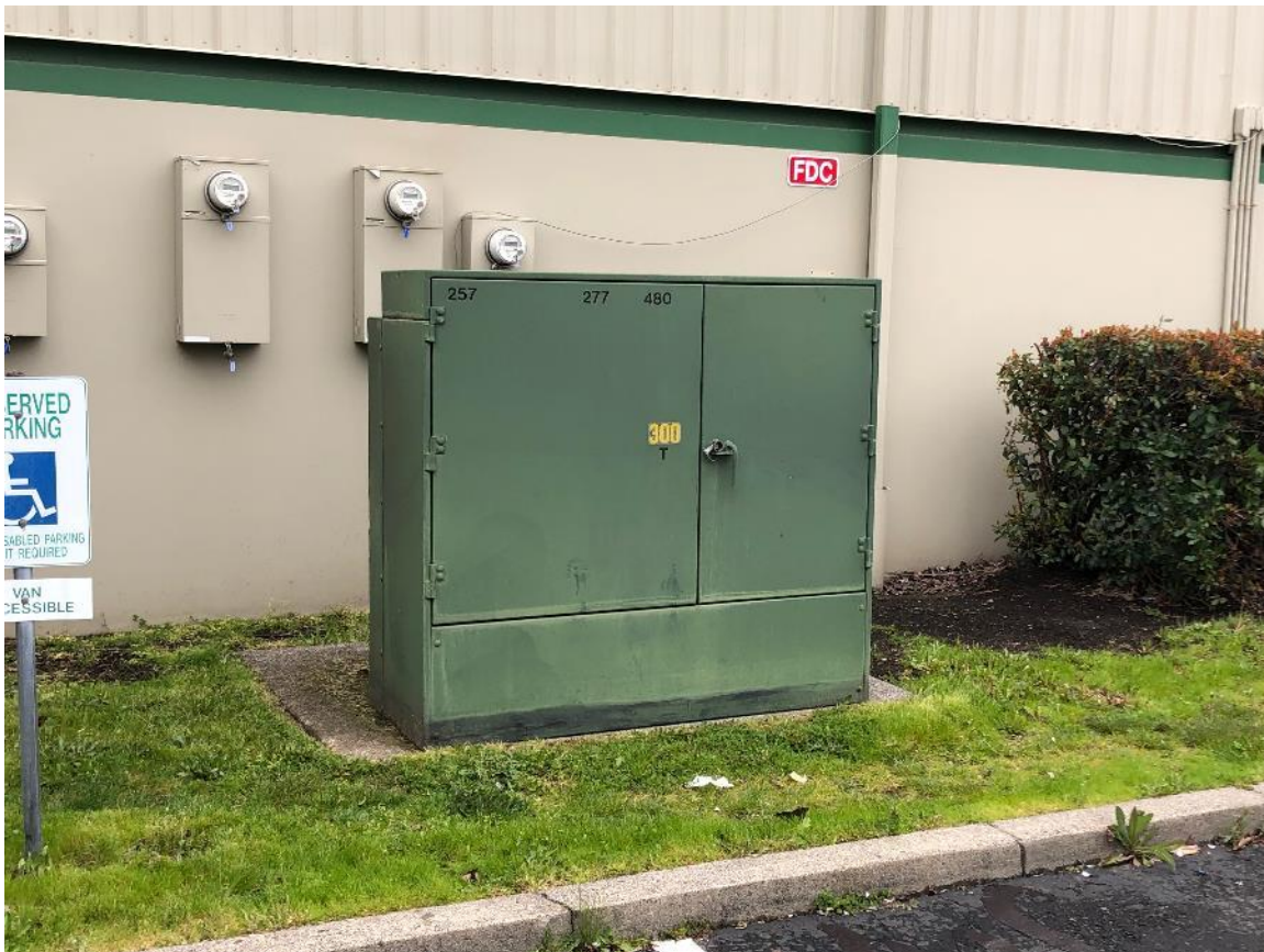
Figure 25: Existing onsite transformer.
