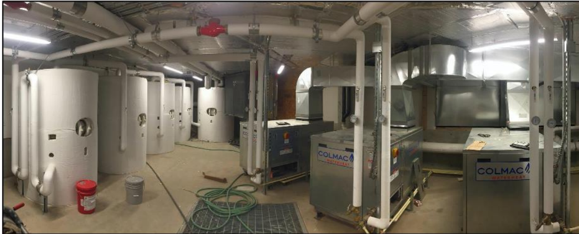
Figure 20: Central HPWH equipment with 2,500 gallons storage located in a parking garage in the Batik Apartments, Seattle, WA. (Courtesy of Ecotope)
