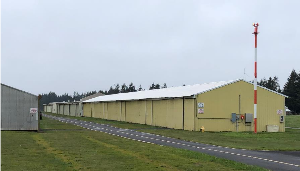
Figure 23: South-facing hangar roofs at Grove Field. An important consideration for using these roofs will be whether the structure can support the additional loads from PV arrays.
