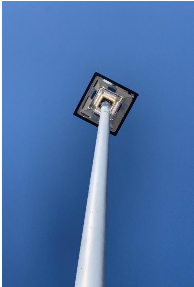
Figure 13: LED site lighting at the Port.
