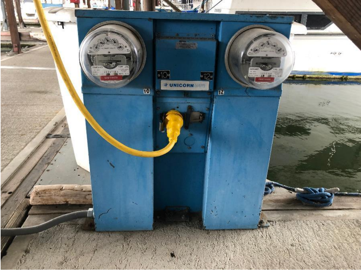
Figure 26: Shore power connection and meter at Parker's Landing.
