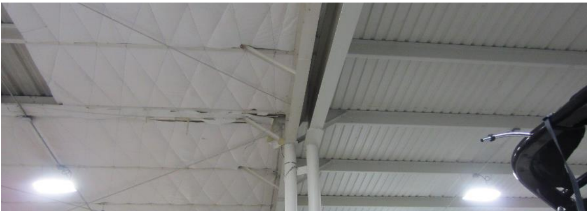
Figure 15: A metal building where part of the building has received an insulation retrofit and part has not.
