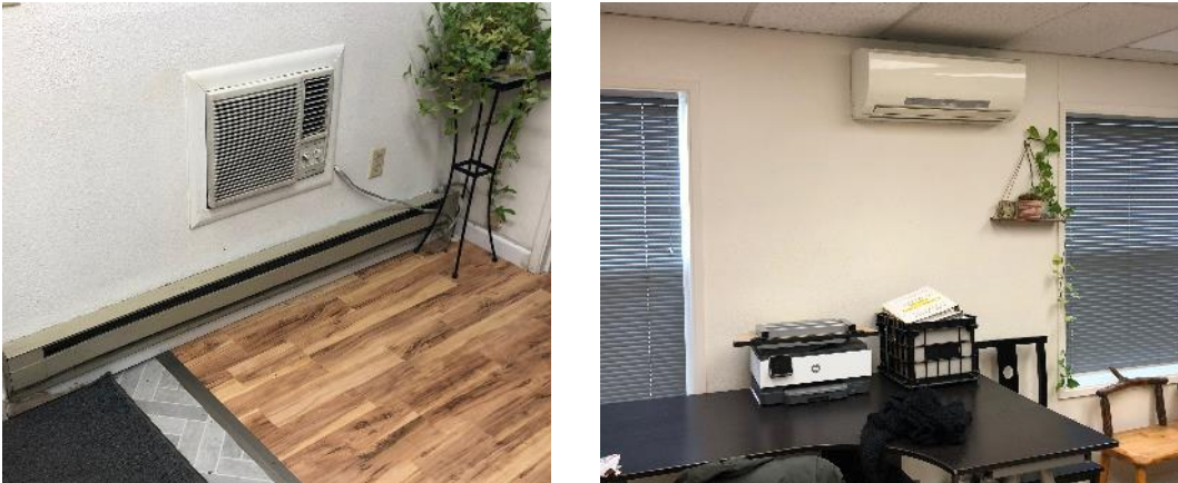
Figure 17: This office space serving a light industrial building originally only had electric resistance heat. Through-the-wall air conditioners were later added for cooling. Both systems have been decommissioned in favor of ductless mini-split heat pumps. The circuits for the resistance baseboard heaters provided enough power for the new heat pumps.
