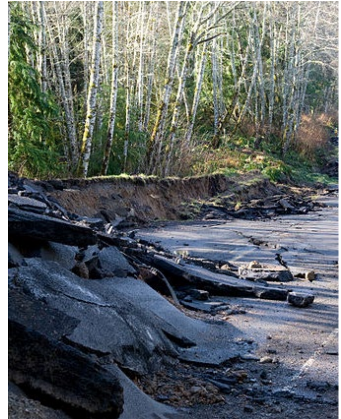
Wikimedia: Flood damaged road, Washington
