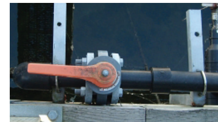
Shutoff at head of docks
