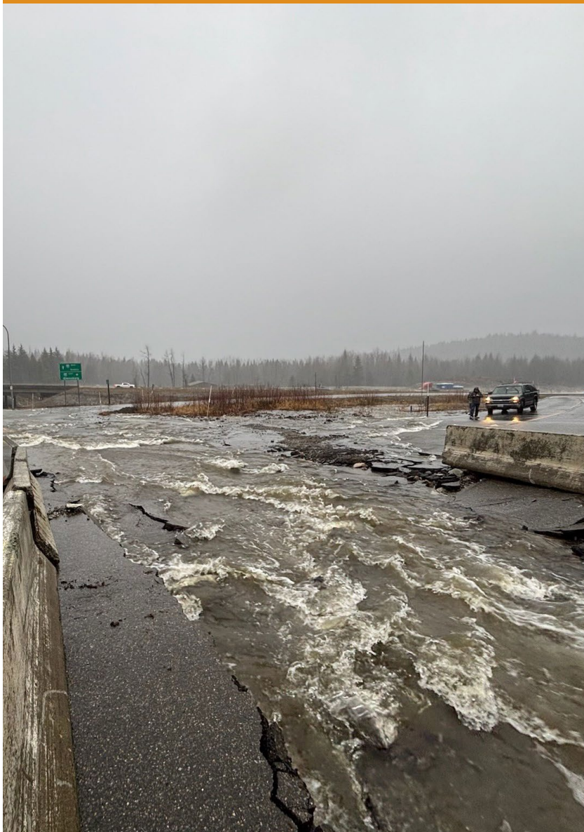
SR 906 wash out near Snoqualmie Pass
