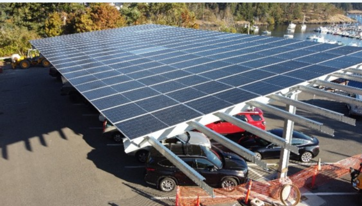
The solar array offers charging and cooling by shading vehicles underneath it. Image courtesy of the Port.
